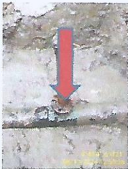
Pic1: Showing one (1no.) 2" flange illegally installed on the pipeline
